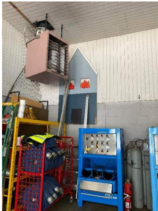
Image 10: Unbraced Suspended Equipment & URM Wall Below Wood Stud Wall "Hinge" Point
